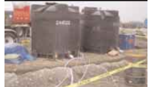
Batch tanks used to prepare injection solutions (e.g., Fe 2+ ), lines then connected to batch tanks
