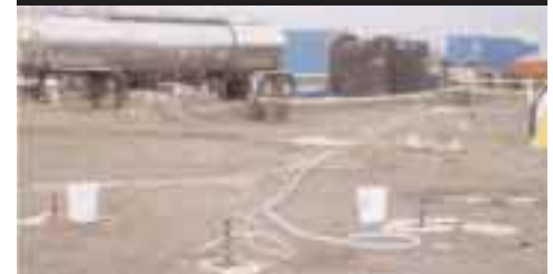
Lines carrying chemicals to injection wells
