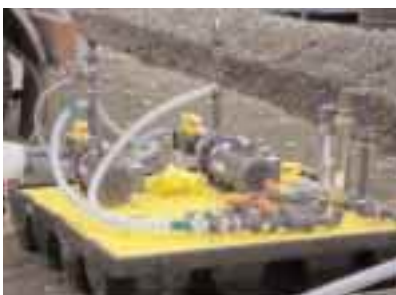
Sulfuric acid injection pump used to acidify aquifer
